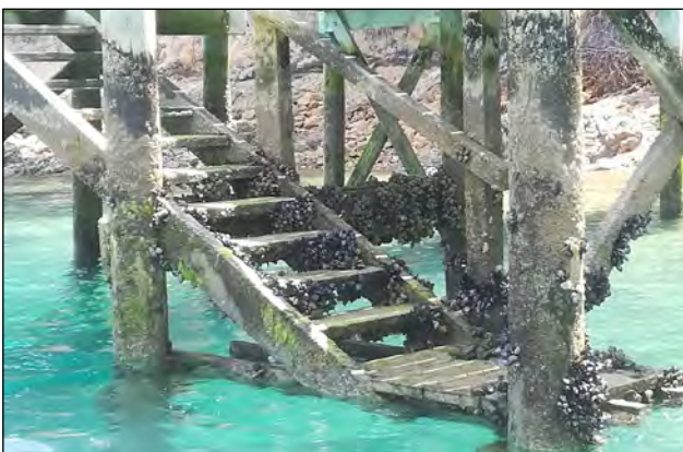
Typical biofouling visible on a jetty at low tide.
