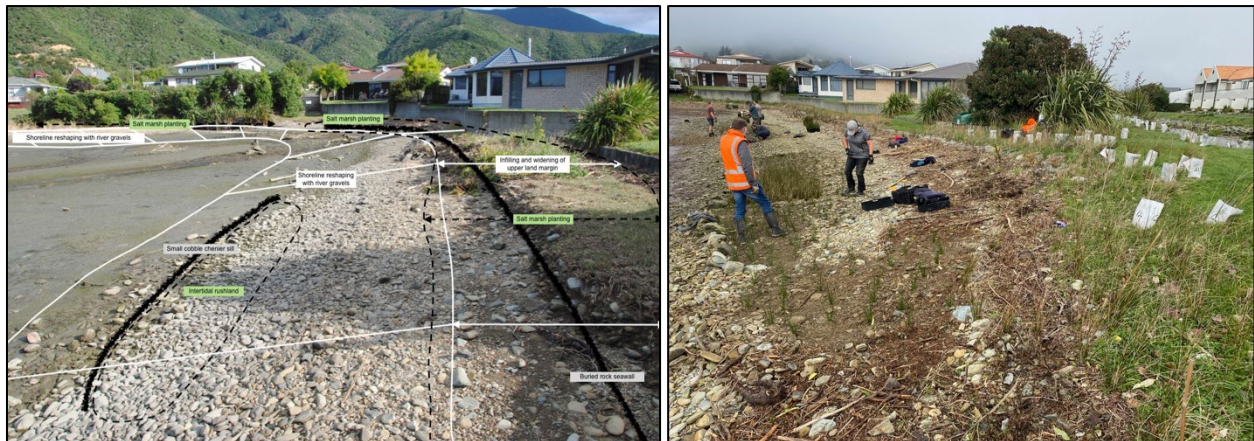
Schematic outline of the restoration area prior to development (left) and post-restoration reshaping and planting (right)
