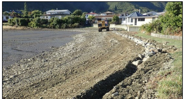
Before and after photos of the primary work site showing the extent of beach replenishment and buried erosion wall
