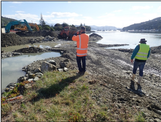
Bunds separated the work site from the estuary to prevent off-site sediment impacts. Stream flow was maintained through a pipe passing through a silt trap (foreground).
