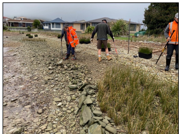
Clearing surface cobbles to create chenier sills and prepare site for planting
