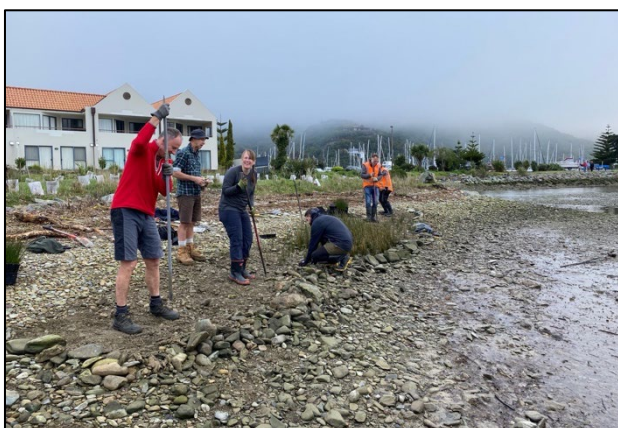
Using crow bars to create deep narrow planting holes behind the rock chenier in the upper intertidal zone
