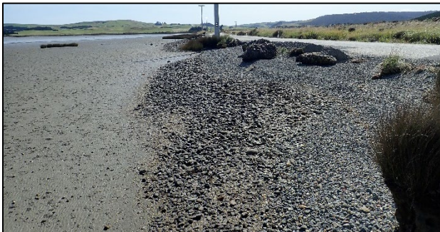
Roading infrastructure disconnecting salt marsh habitat from the estuary, Haldane Estuary, Southland
